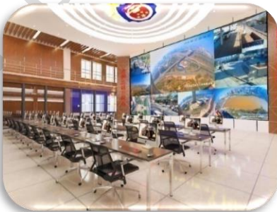
Traffic Control Center
