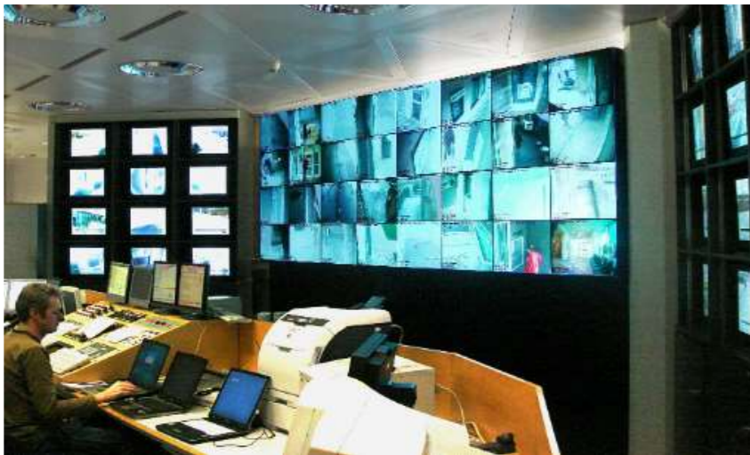
Security Operations Centers video surveillance, monitoring of infrastructure
