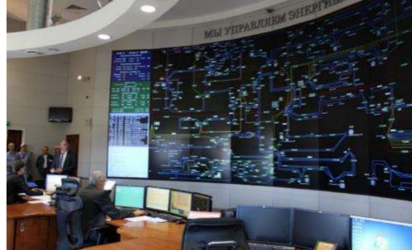
Command and Control Centers: monitoring and management of processes in energy, transport, telecommunications sectors, NOC
